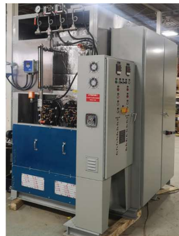
960 kW @ 480 V Steam Boiler for Ferguson Enterprises, Newport, VA, USA
